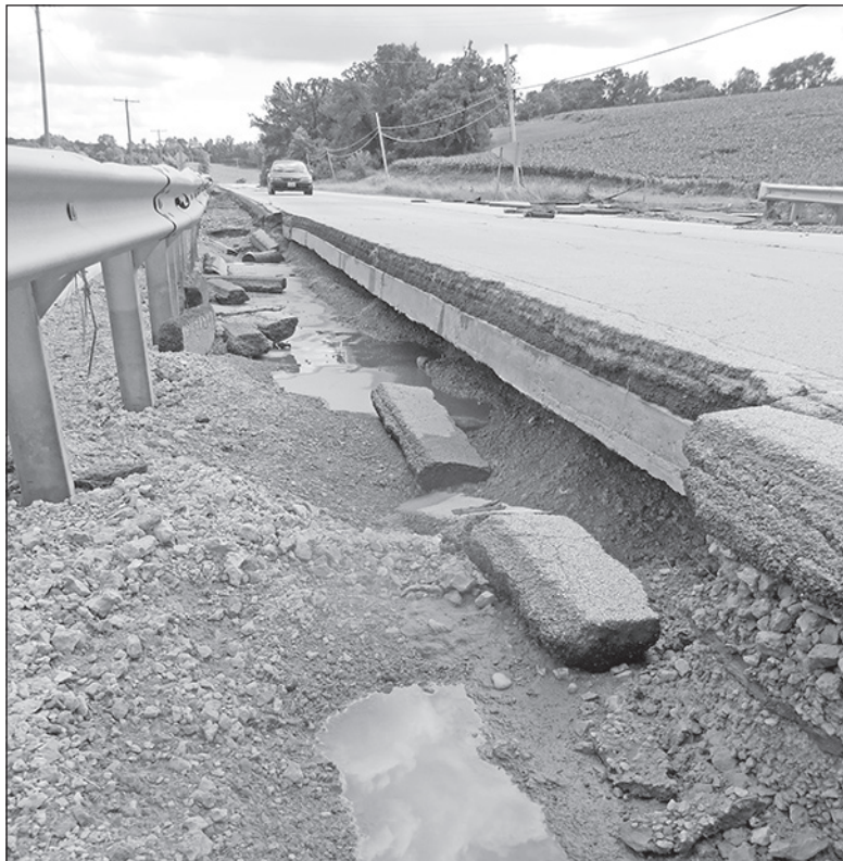
This section of the road at Louisa Road and Hwy 73 north of Lena is underlain by a box culvert that when installed was covered first with a layer of gravel, then cement, then blacktop. The gravel washed out from under the road leaving it unsupported, actually suspended. The road is closed indefinitely.
