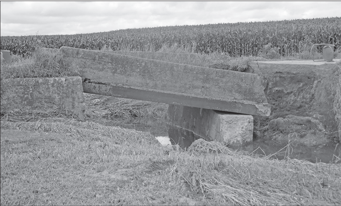
This bridge is on a private drive just south of Lena on Hwy 73. The footings are completely washed away.
